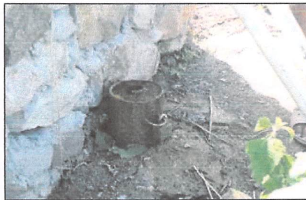
Figure 3. Water overflows in SP.4
